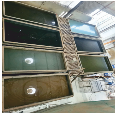
7 Tank Pre Treatment Plant
